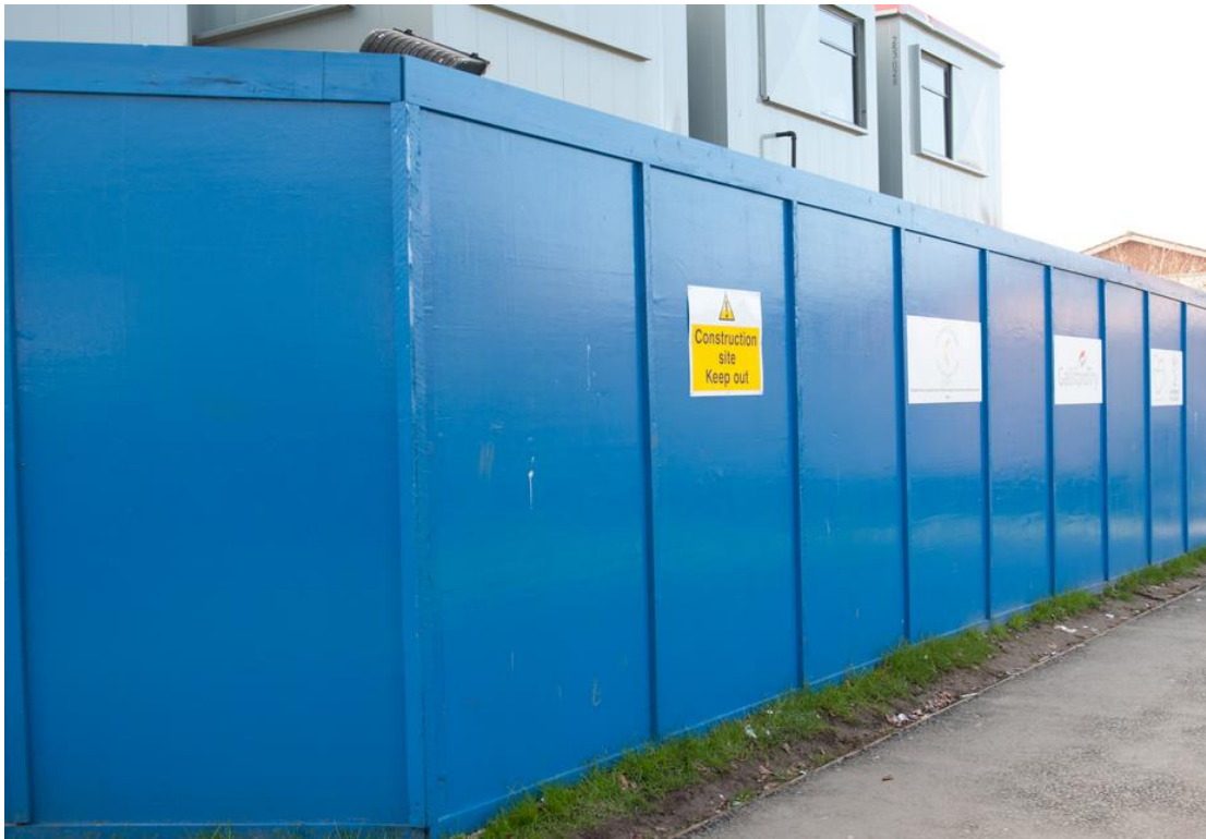
Figure 3 Example of hoarding to be used on site perimeter (which may include graphics of the proposed development)
